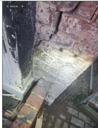
Photograph 3: Main crevice on corner of front elevation
